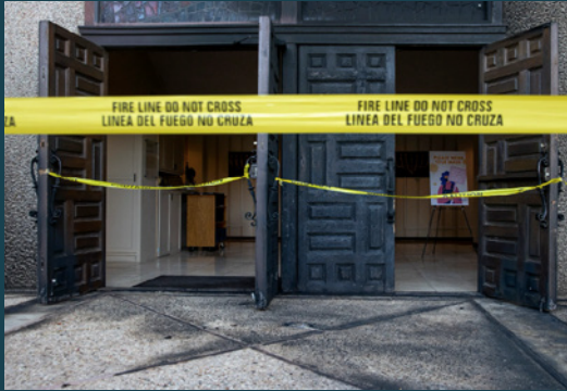
Fire and smoke damage at Congregation Beth Israel - Austin
